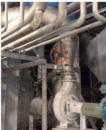
Figure 4. TCR-2501 total consistency transmitter installed after a pulper
