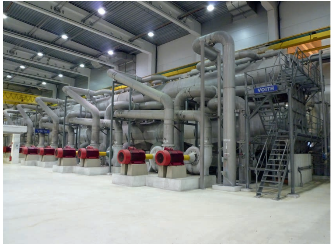
Figure 1. Flotation cells in the DIP plant of UPM Hürth, Rhein Papier GmbH
