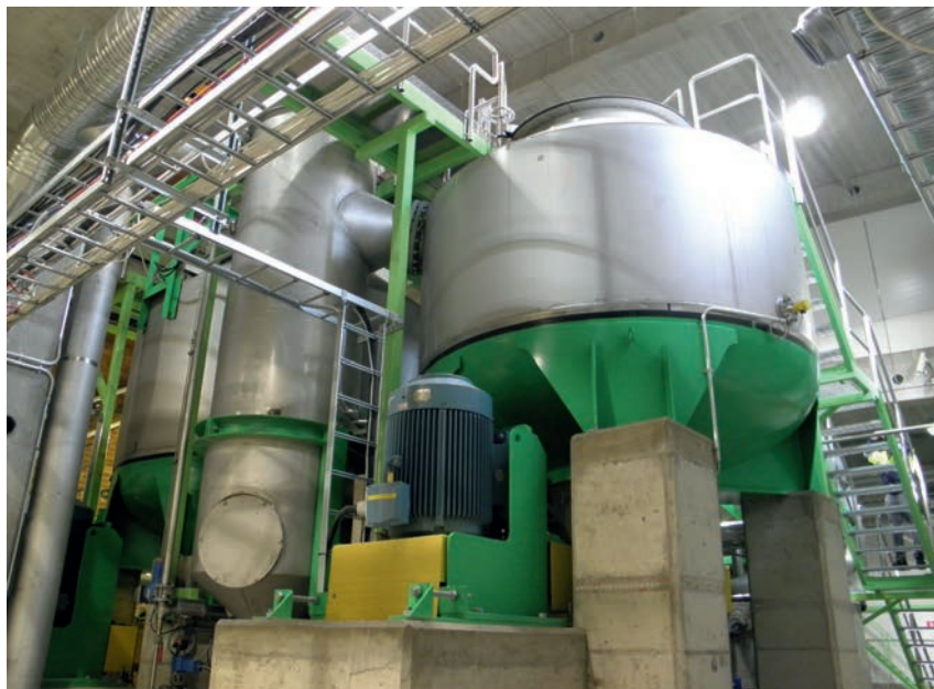
Clarifier and secondary pulper, GL&V
