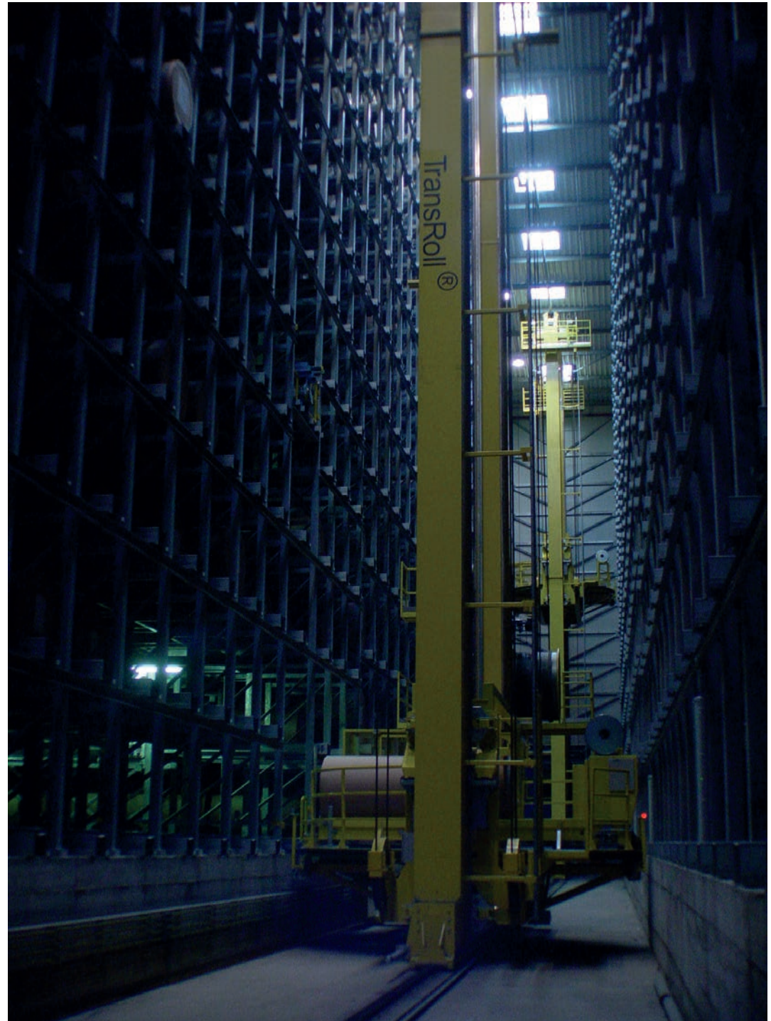
Figure 1 TransRoll stacker cranes between the rack structure, and the channel vehicle at the first level ready to deliver roll set on the out take conveyor
